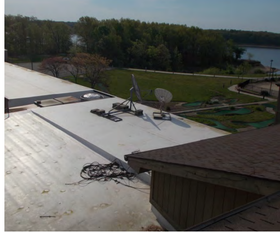
Figure 72- Existing Cable TV Dish Antennae
