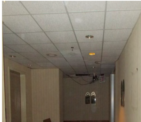
Figure 78 - Existing PA Speaker - Corridor
