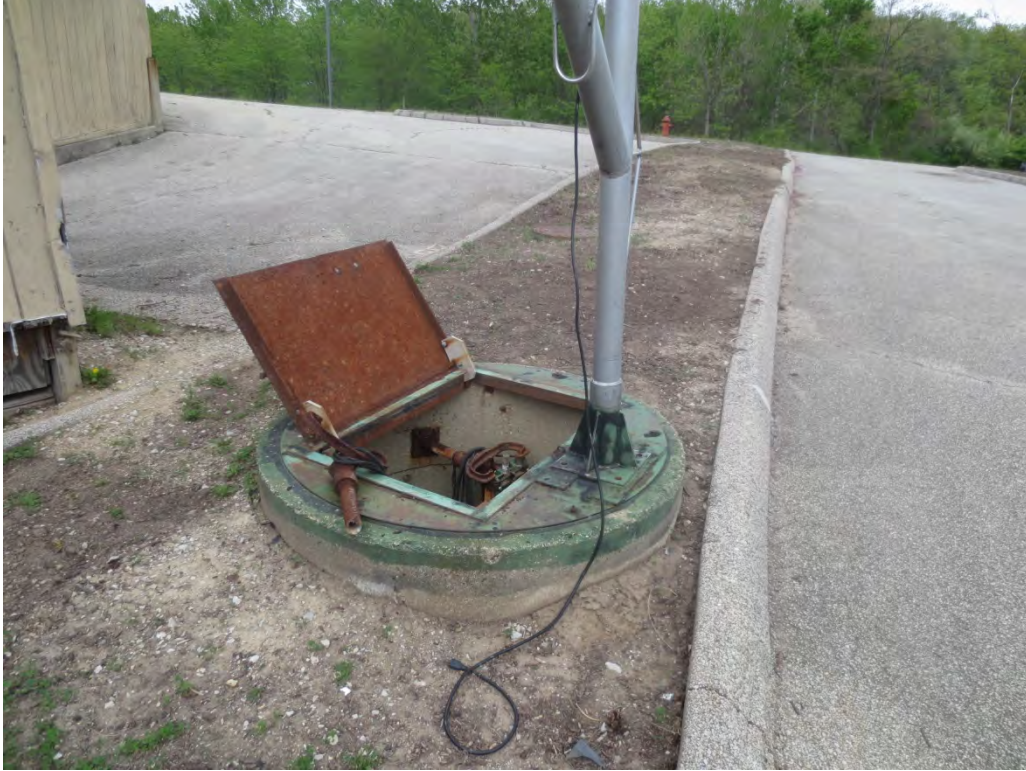
Sanitary Sewage Pump Station near dock area
