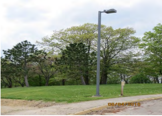
Figure 51 - Typical 30'-0" Pole Lighting
