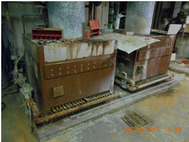
Figure 2 – Hot water boilers
