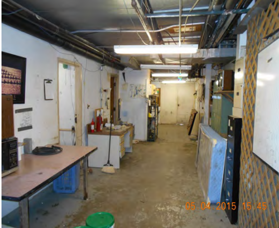
Figure 15 – Utility room corridor lighting
