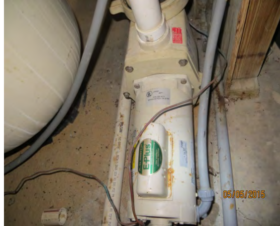
Figure 14 – Water pump for spa
