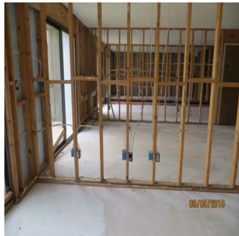
Figure 63 - Typical Guestroom with Back-to-Back Telephone Outlets with Coiled Telephone Wires
