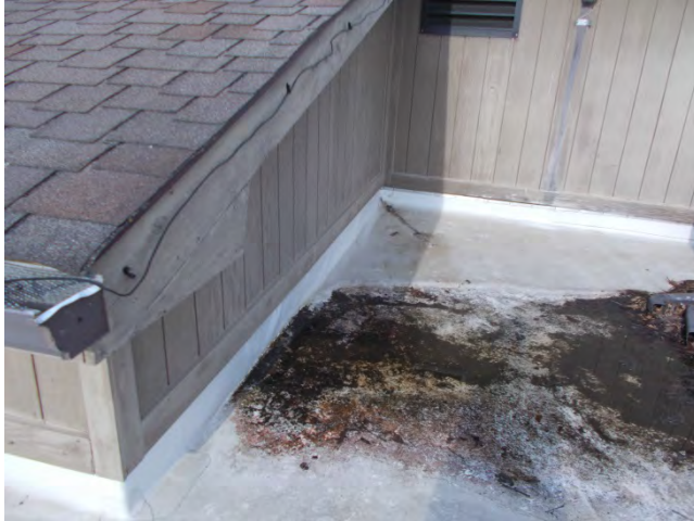
Figure 27 – Mold at Flat Roof
