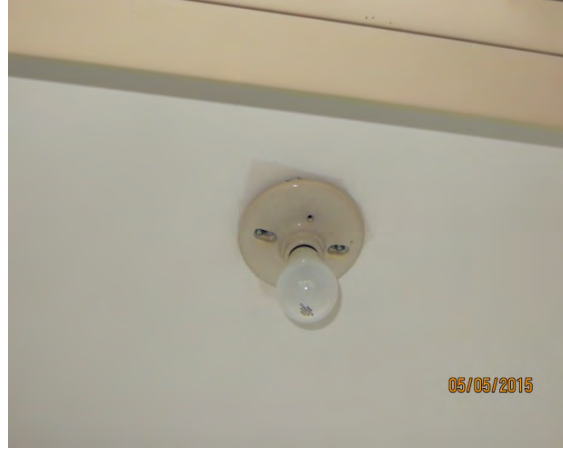
Figure 48 - Typical Suite Closet Light
