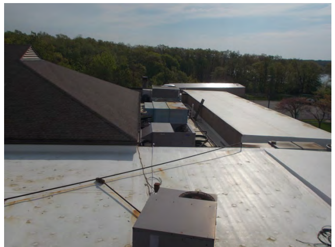
Figure 18 – Mechanical Equipment on Flat Roof
