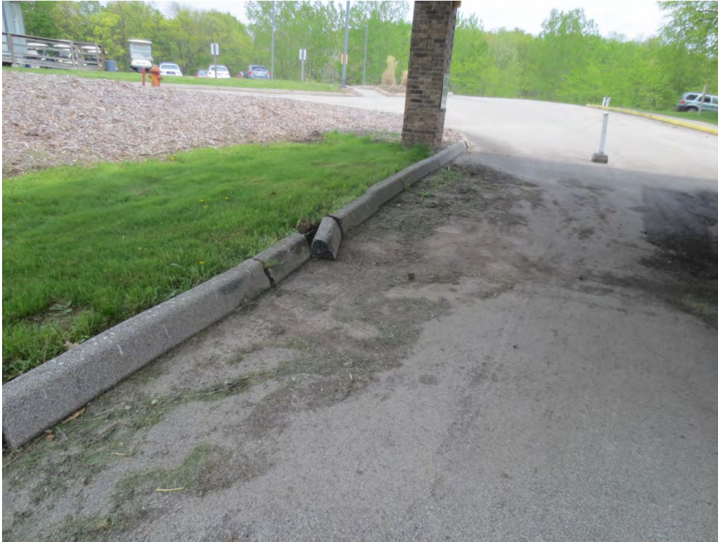
Asphalt curb cracks / displacement at entrance
