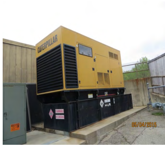
Figure 2 - 750kW Diesel Generator
