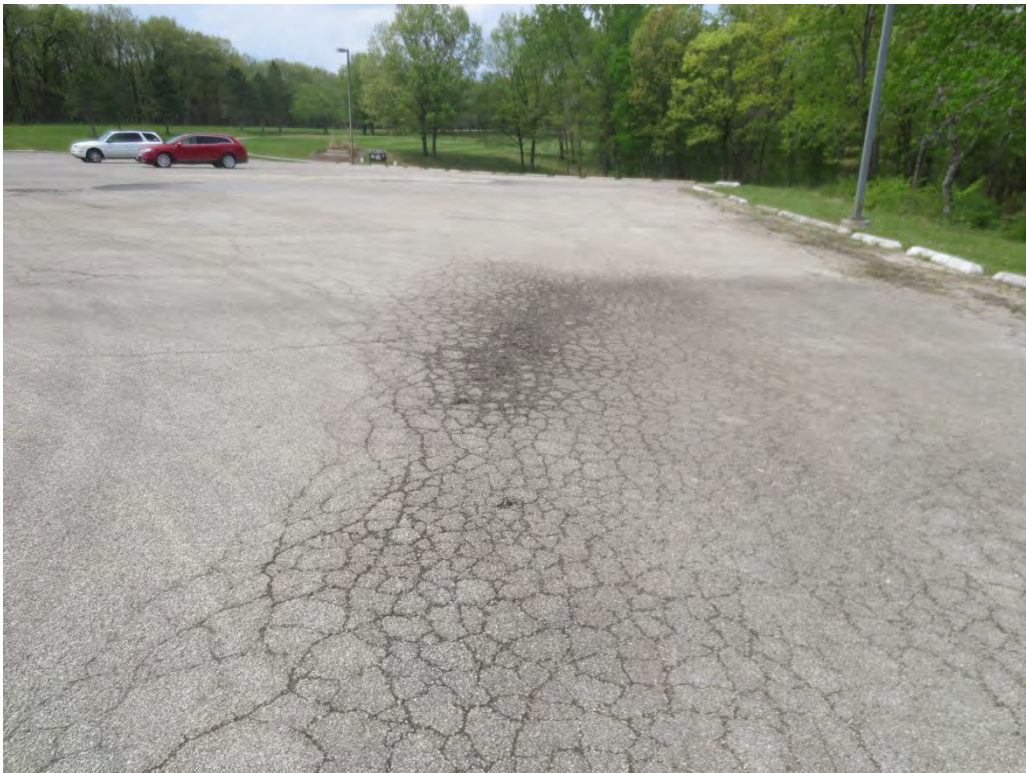
Evidence of localized ponding and pavement deterioration
