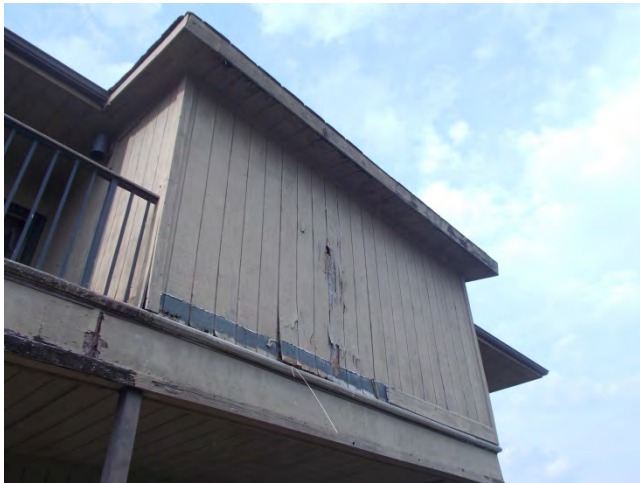
Figure 7 – Typical Wall Deterioration
