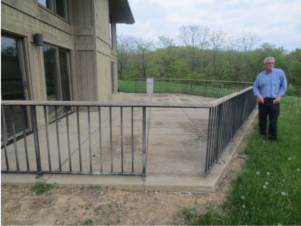
Patio and railing at rear of Eagle's Landing (Note missing guardrail)
