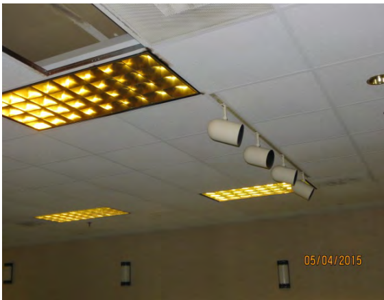
Figure 31 – Lounge area lighting
