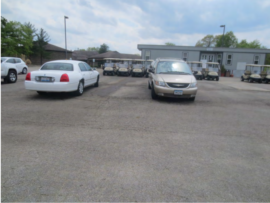
Parking by temporary Pro Shop – two ADA spaces to left of carts, significant alligator cracking
