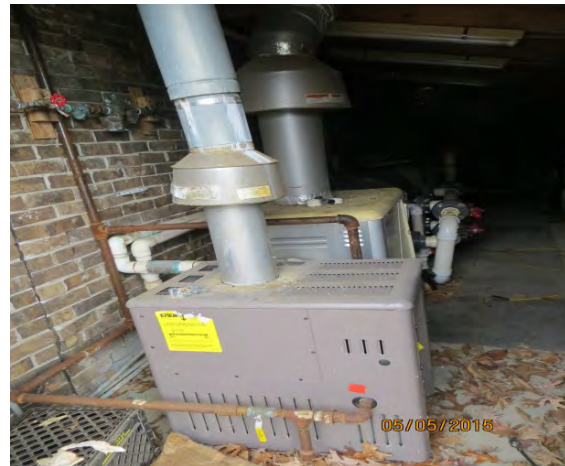
Figure 12 – Swimming pool water heater
