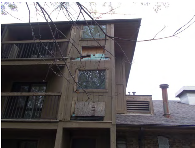
Figure 9 – Exposed A/C Openings in Wall
