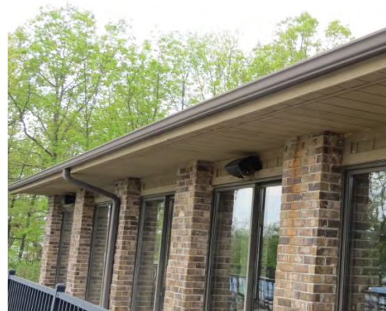
Figure 80 - Existing PA Speaker – Perimeter
