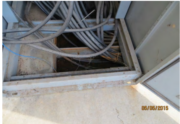
Figure 6 – 2500 amp, 277/480VAC main switchboard with submerged service feeders
