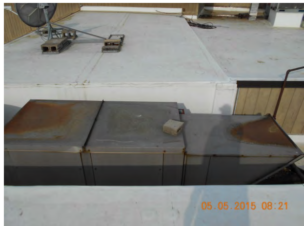
Figure 6 – Kitchen and coffee shop makeup air unit
