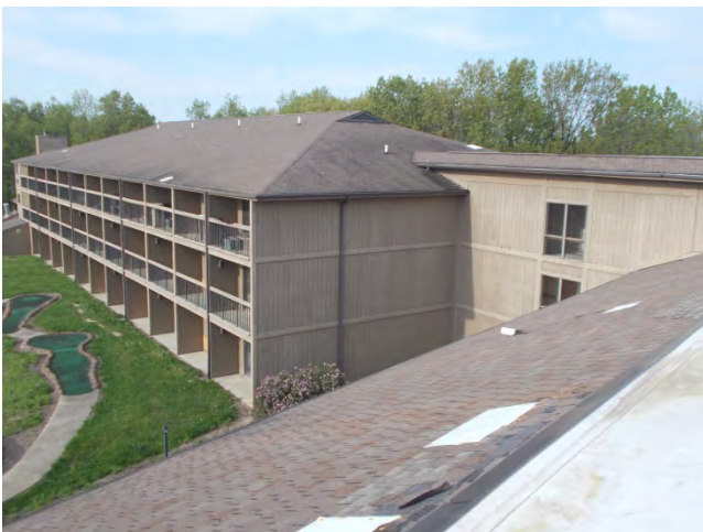
Figure 17 – Shingled Roof (Note Roof Patches)
