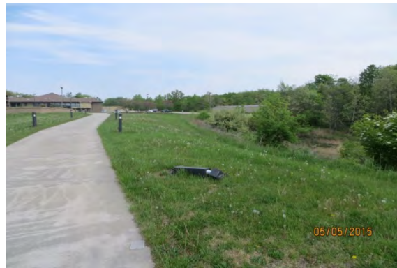
Figure 54 - Bollard Fixture Rooted-up
