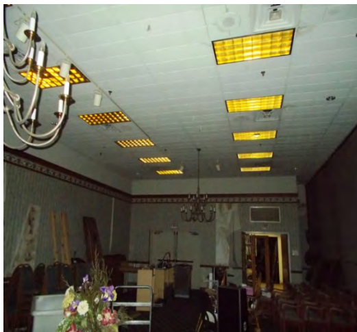
Figure 79 - Existing PA Speaker – Restaurant
