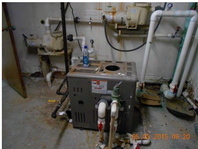
Figure 12 – Indoor pool gas fired water heater
