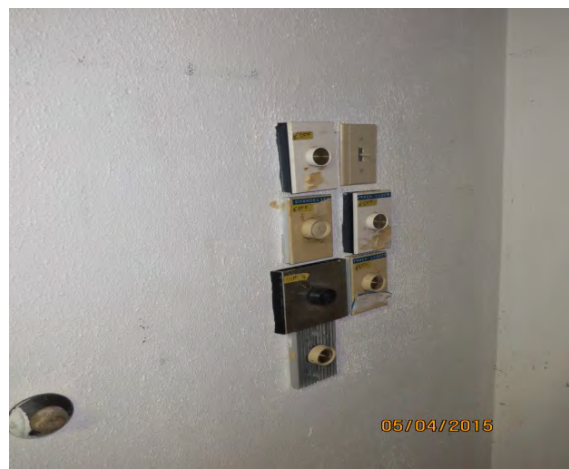
Figure 26 – Banquet area rotary dimmer switches
