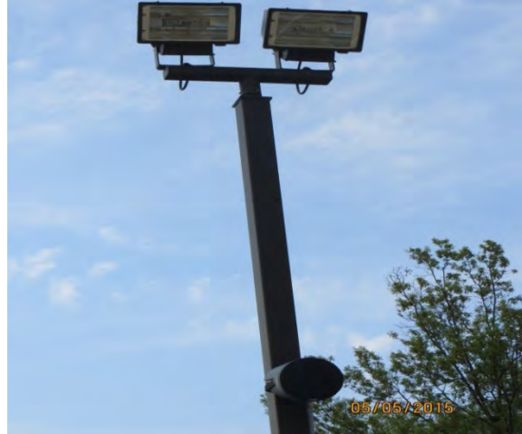
Figure 82 - Existing PA Speaker – Outdoor Swimming Pool Area
