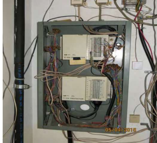
Figure 61 - Existing Telephone Hub Panel
