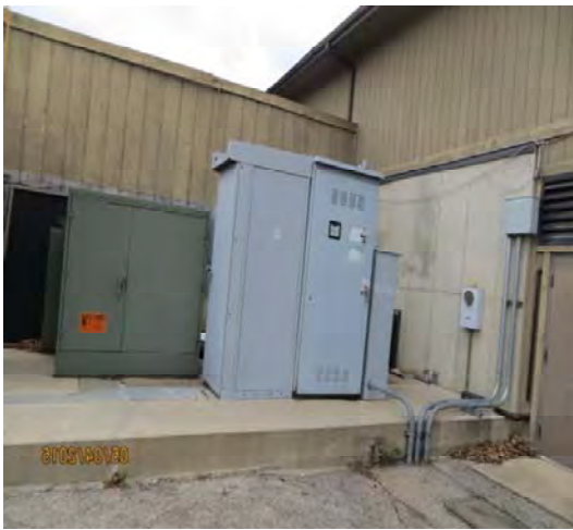
Figure 1 – Utility transformer and automatic transfer switch
