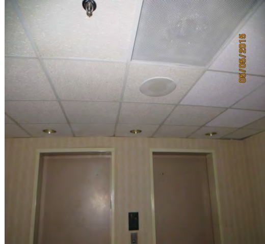
Figure 76 - Existing PA Speaker – Lobby
