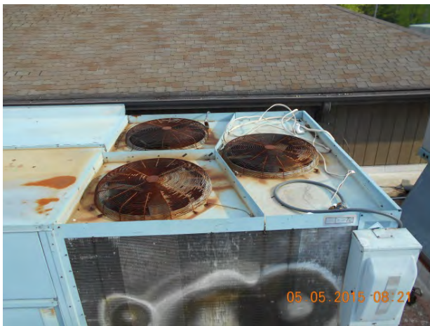
Figure 5 – Restaurant and bar/lounge mechanical rooftop unit
