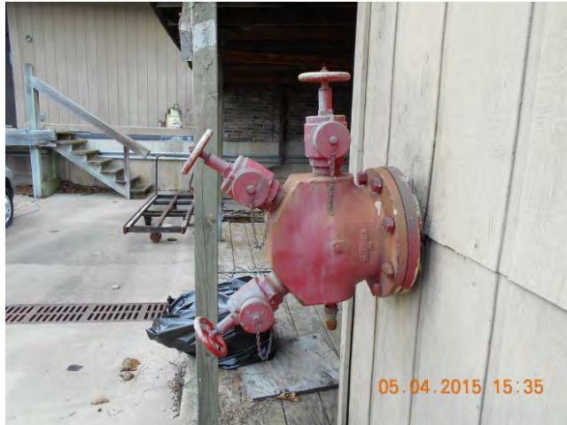
Figure 3 – Fire department test header
