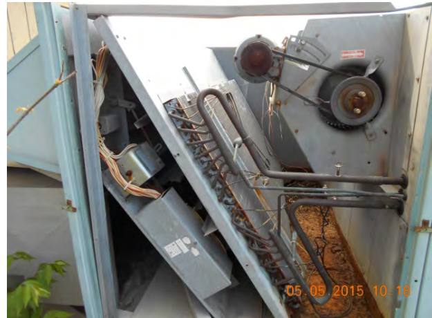
Figure 8 – Eagle's Landing air handling unit
