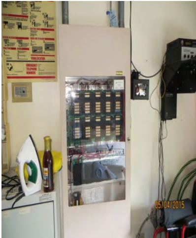
Figure 65 - Existing Main Fire Alarm Panel
