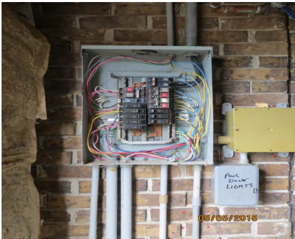
Figure 11 –Outdoor swimming pool panelboard
