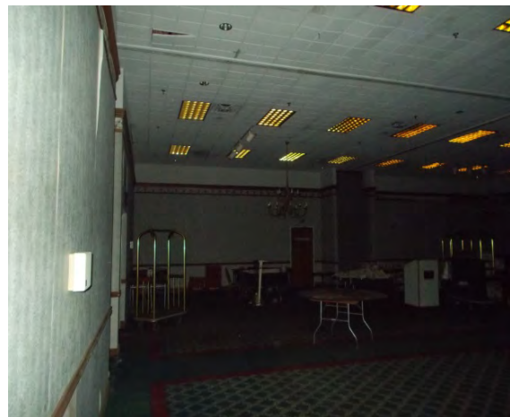
Figure 24 – Banquet areas: pendant and recessed lighting fixtures
