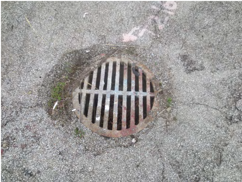
Debris filled catch basin adjacent to backup generator
