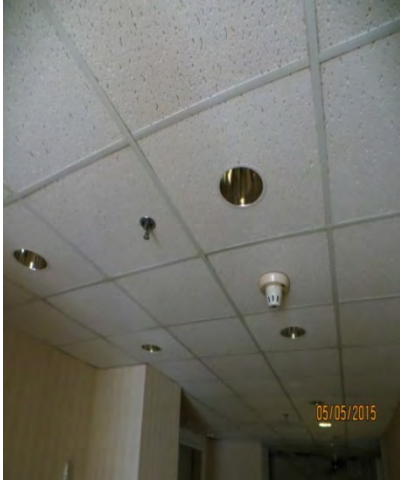
Figure 67 - Existing Smoke Detector Adjacent To Elevator Lobby
