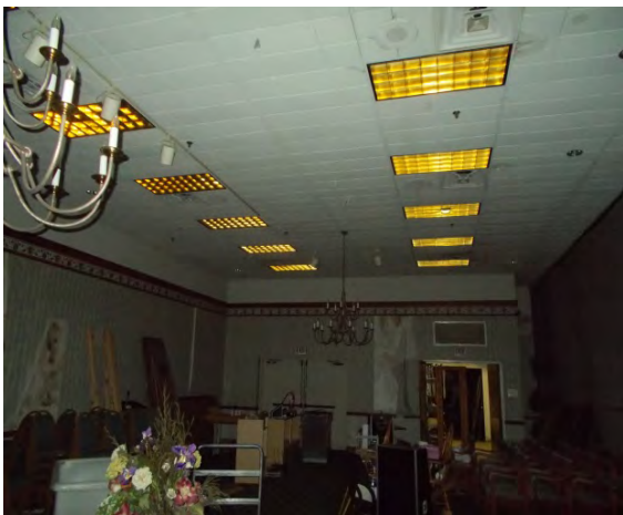
Figure 23 – Banquet areas: pendant and recessed lighting fixtures
