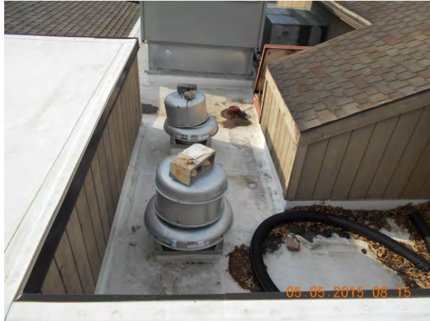
Figure 9 – Rooftop exhaust fans
