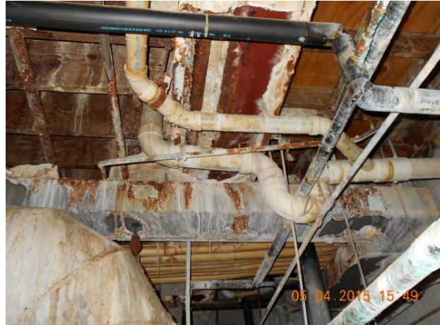
Figure 10 – Mechanical room ductwork corrosion
