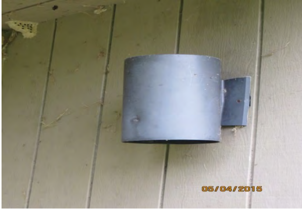
Figure 57 - Building Perimeter Incandescent Wall Sconces
