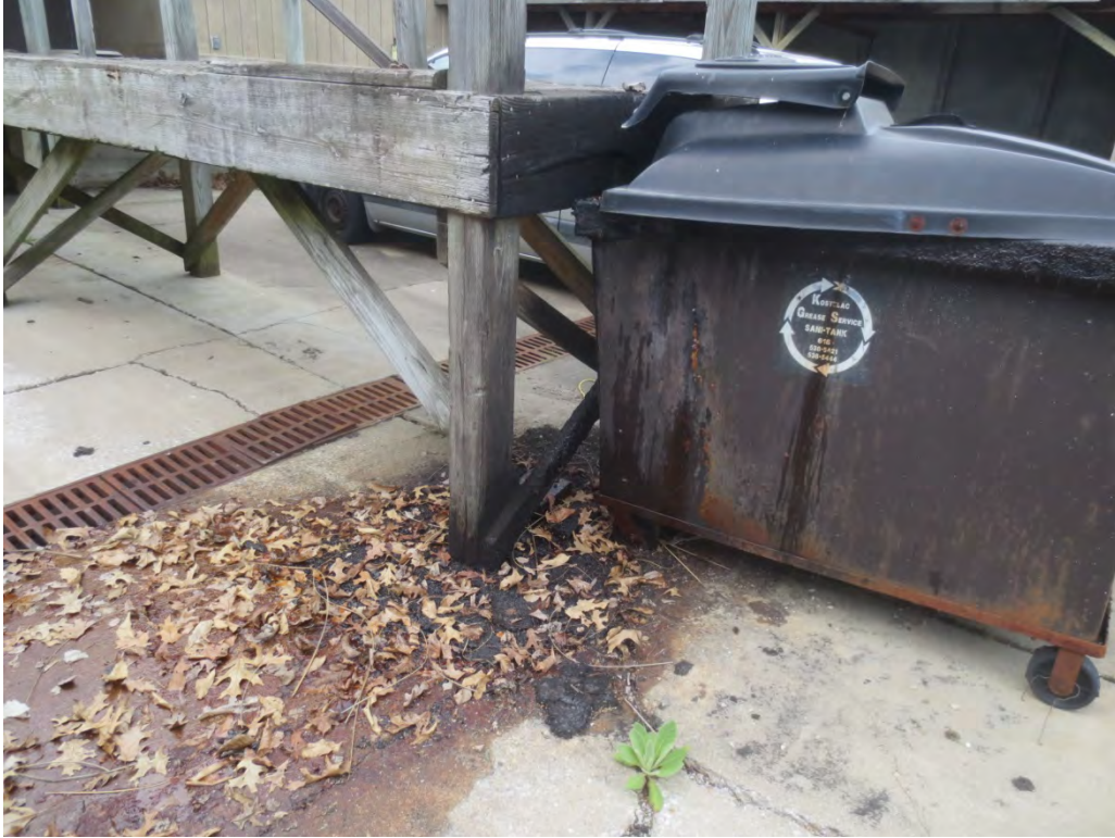
Leaking grease tank draining to storm drain
