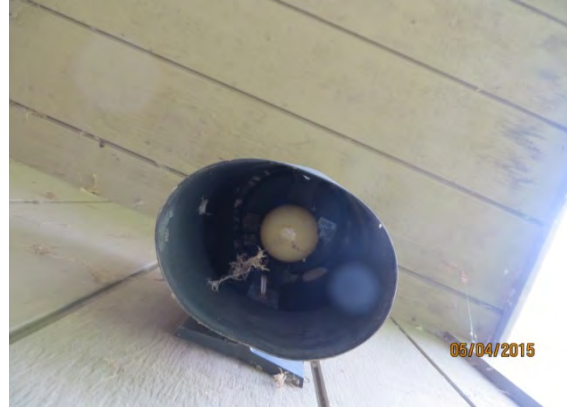
Figure 58 - Building Perimeter Incandescent Wall Sconces
