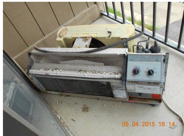
Figure 2 – Guestroom PTAC unit stored on balcony
