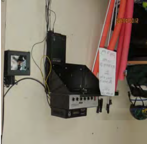
Figure 75 - Existing Main PA System
