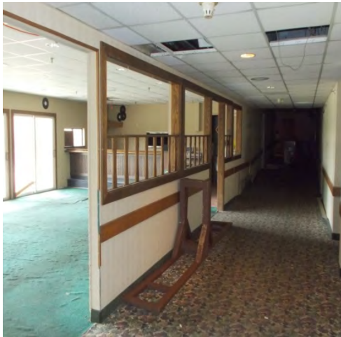
Figure 77 - Existing PA Speaker - Corridor
