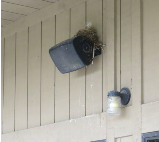
Figure 81 - Existing PA Speaker – Outdoor Swimming Pool Area
