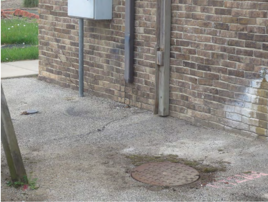
Roof drain discharging to pavement
