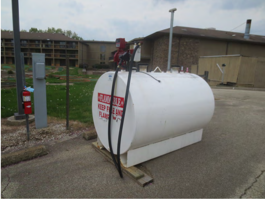
Unprotected fuel tank adjacent to mini-golf
