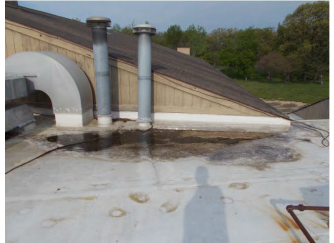
Figure 28 – Ponding at Flat Roof
