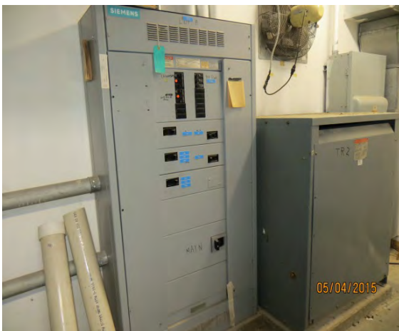
Figure 7 – First floor electrical room
