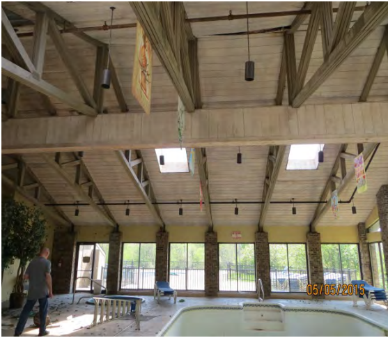
Figure 39 – Pendant incandescent lighting fixtures
