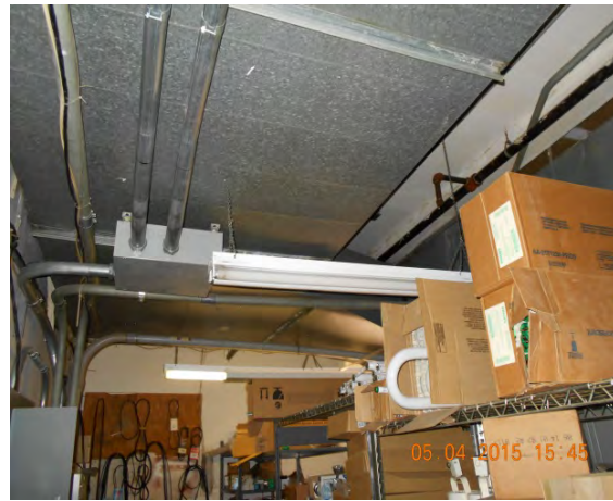
Figure 18 – Main switchboard room lighting
