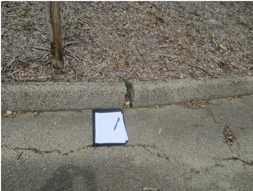
Asphalt curb cracks - typical
