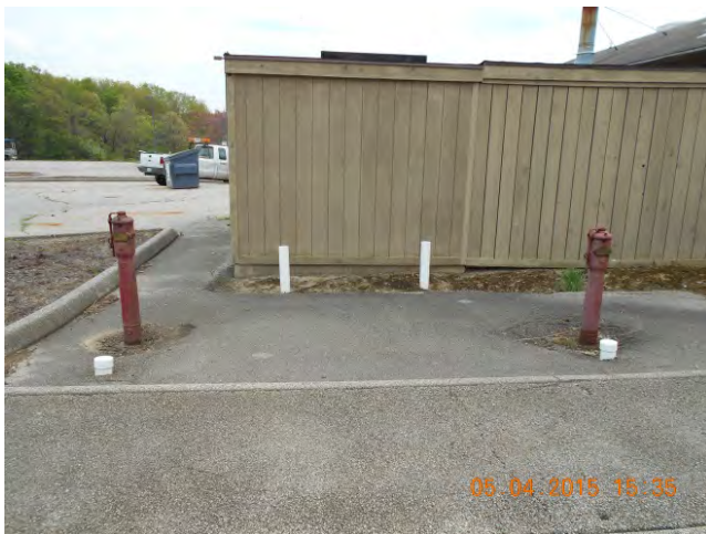
Figure 1 – Post indicator valves located above underground water tanks
