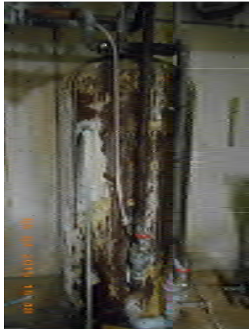
Figure 3 – Domestic water surge tanks
