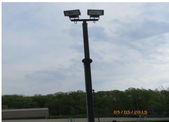
Figure 55 - Typical Outdoor Swimming Pool Flood Light HID Fixtures Building perimeter wall mounted fixtures need to be replaced (Figures 57 and 58).
