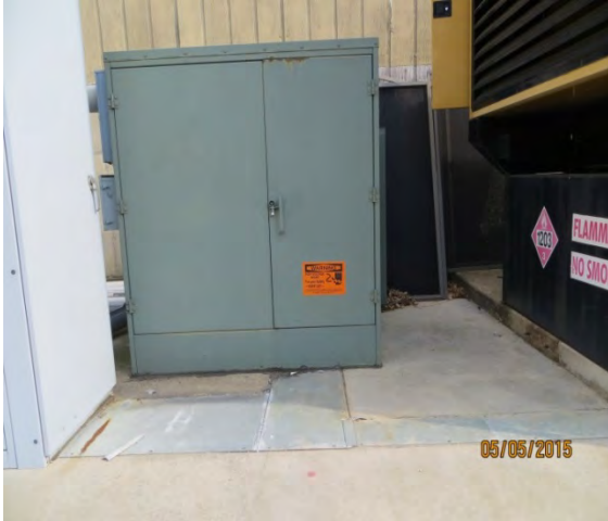
Figure 3 – Metal trench with service feeder cables
